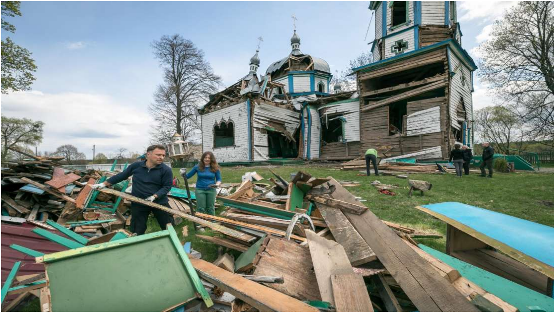
On the ground damage assessments and salvaging
